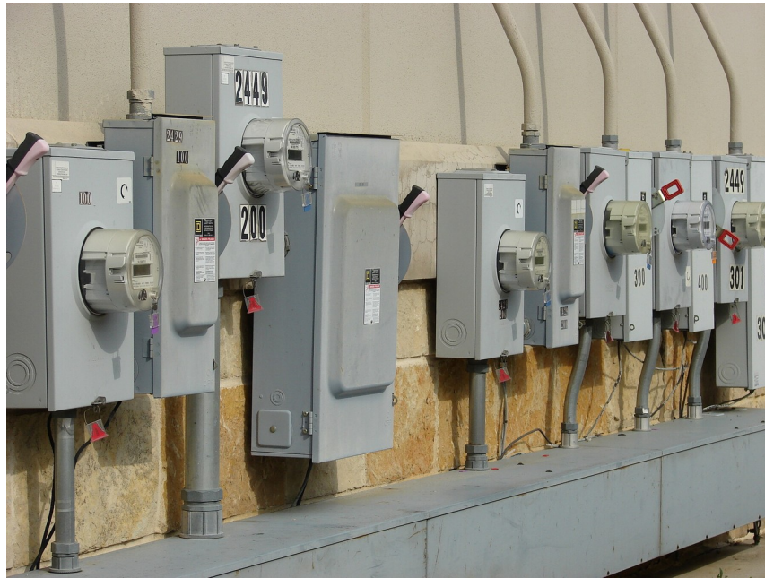
Figure A-3 - Outdoor meters and service enclosures
