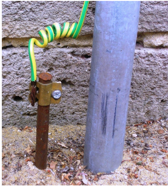
Figure A-8 - Grounding electrode installation used as an error-spotting exercise
