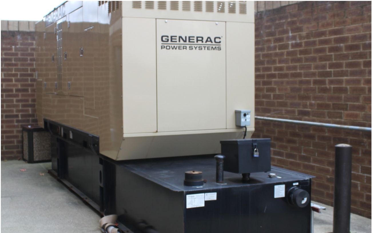
Figure 11-1 - Outdoor commercial standby generator
