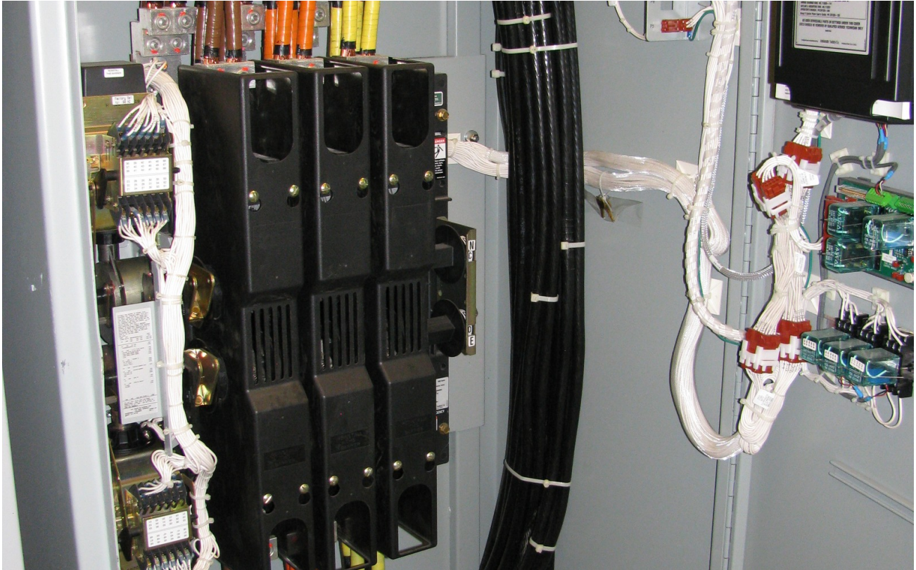
Figure 11-2 - Large automatic transfer-switch assembly
