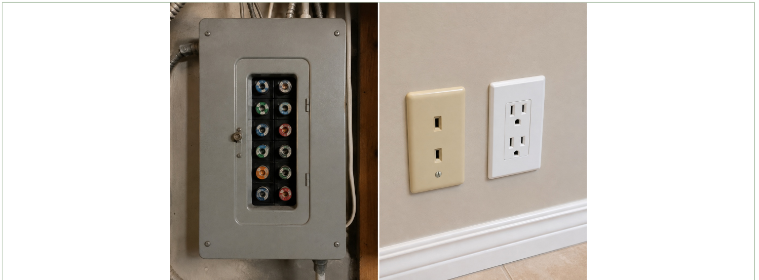
Left: fuse panel. Right: older two-slot and modern three-slot receptacles.
