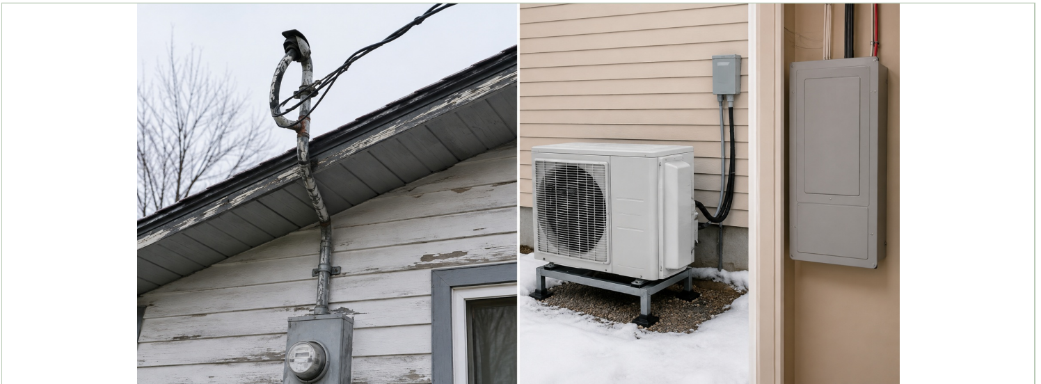
Left: weathered service entrance. Right: heat pump, disconnect, and closed panel.
