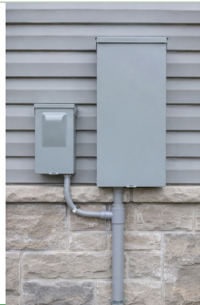
Approved transfer equipment prevents unsafe backfeed.
