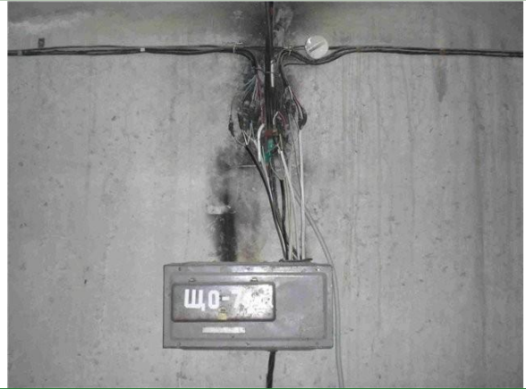
Hidden damage can be severe. Water, contamination and deteriorated connections require professional evaluation - not surface drying.
