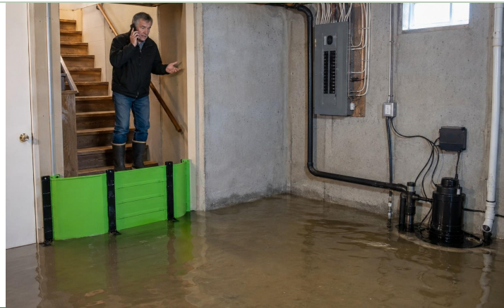
Stay out of floodwater and away from panels, receptacles and connected equipment.
