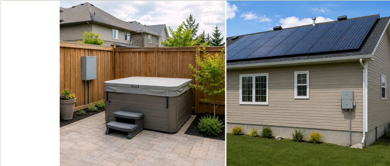
Left: hot tub and nearby electrical equipment. Right: rooftop solar system.
