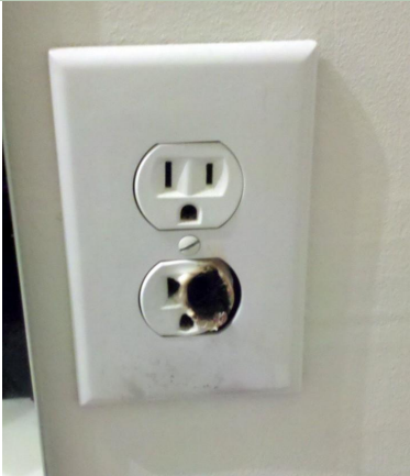
Scorching means stop using the receptacle and arrange an assessment.
