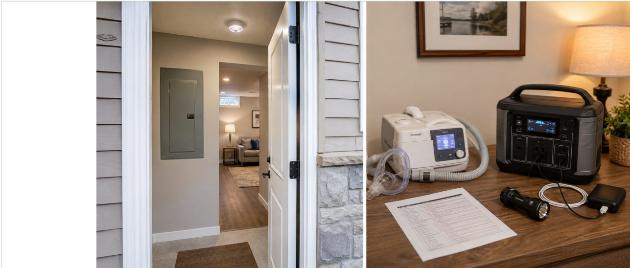
Left: panel serving a secondary living space. Right: medical device and portable backup power.
